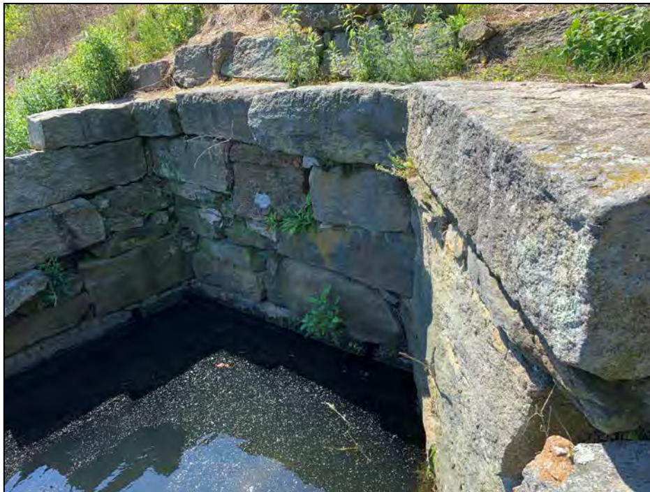
Photo No. 28: Outlet end and downstream headwall for the low-level outlet conduit.
