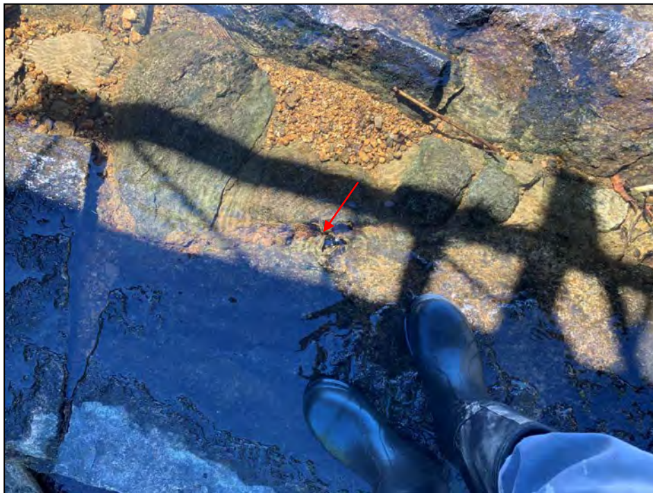
Photo No. 22: Vortexing (arrow) of leakage flow through the open masonry of the control section.
