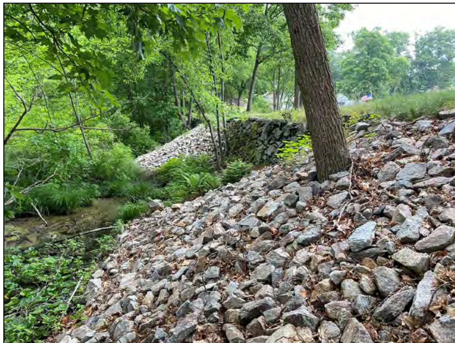
Photo No. 36: Downstream side of the dike from near the tallest section looking right. Note the two trap rock buttresses and ponded water within the downstream area.
