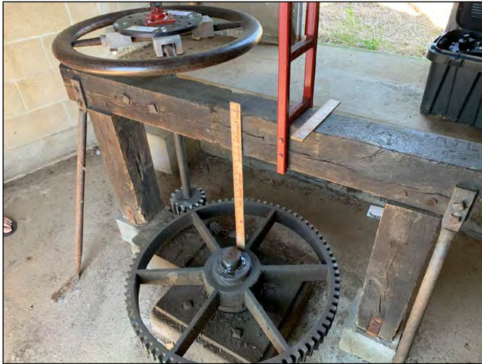
Photo No. 27: Gate operator for the low-level outlet system.
