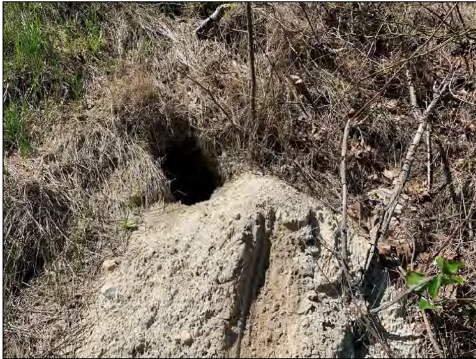
Photo No. 17: View of one of the burrows. Note diameter (12 inches) and soil spoil pile (silty fine sand) typical of all four apparent burrow locations.
