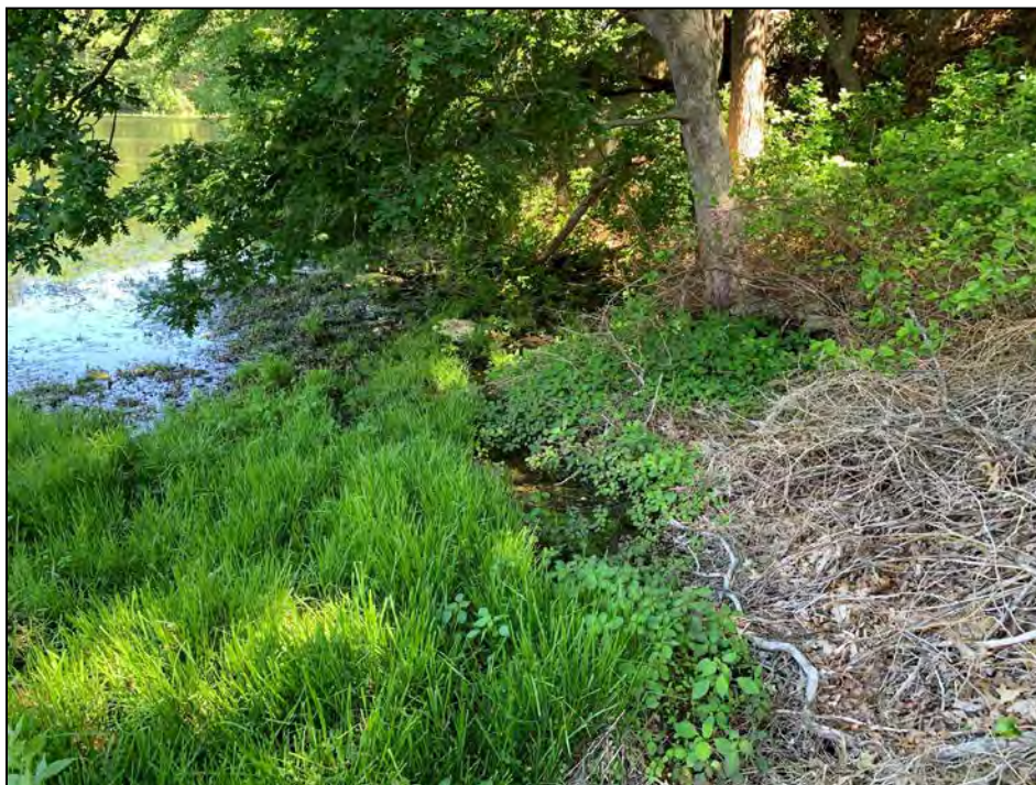
Photo No. 19: Apparent seepage area at the toe of the right groin of the downstream slope.
