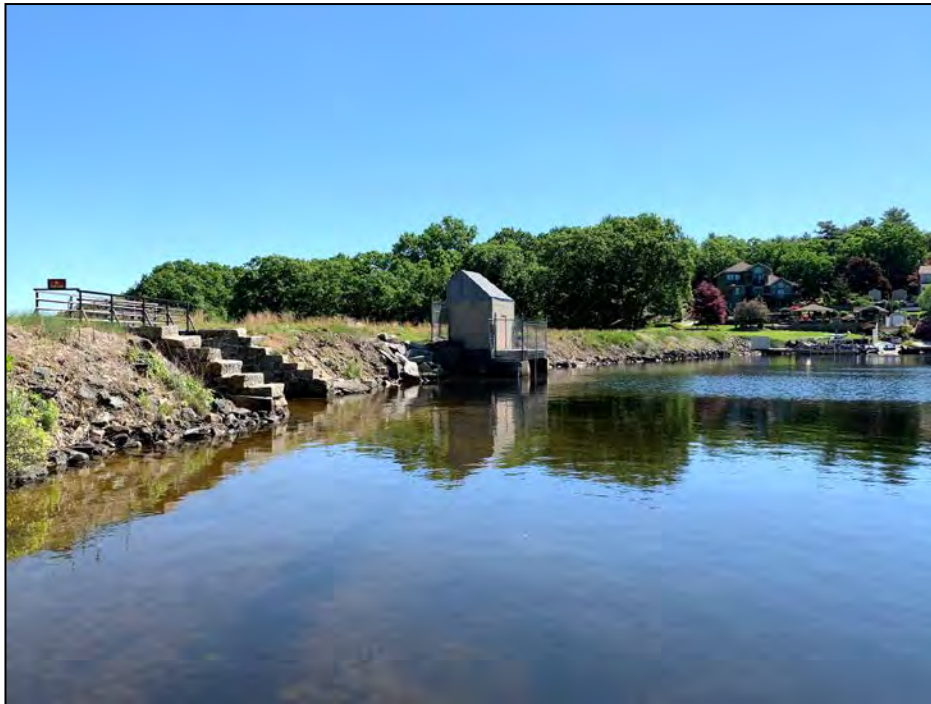
Photo No. 1: Overview of the upstream face of the dam from the left abutment.
