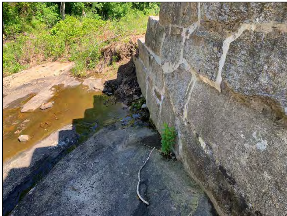
Photo No. 24: Leakage through the base of the downstream right training wall approximately 20 feet downstream of the control section.
