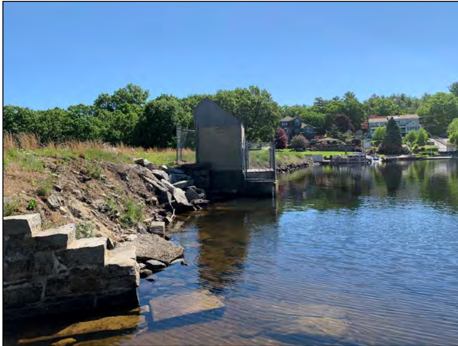
Photo No. 5: Upstream slope between the spillway and low-level outlet. Note bare soil along top of slope.
