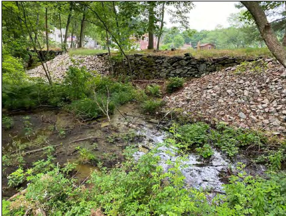
Photo No. 37: View of the tallest section of the downstream side from 50 feet downstream looking upstream.
