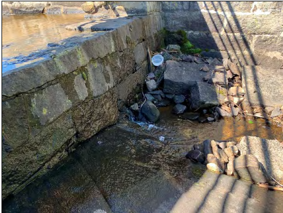
Photo No. 23: Leakage through the spillway control section.
