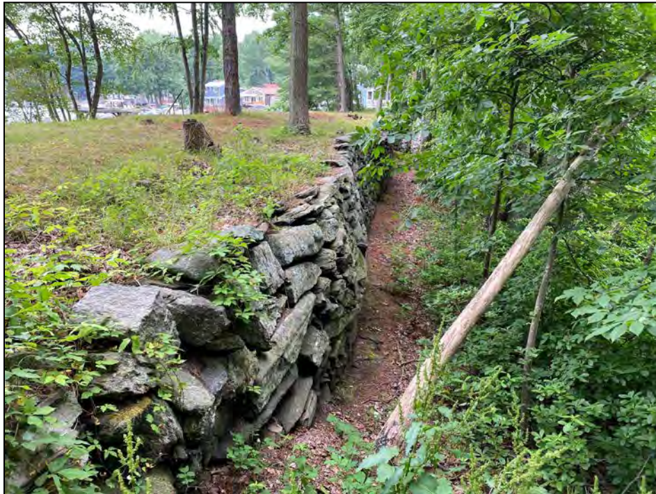
Photo No. 35: Downstream side of the dike from the right abutment looking left.
