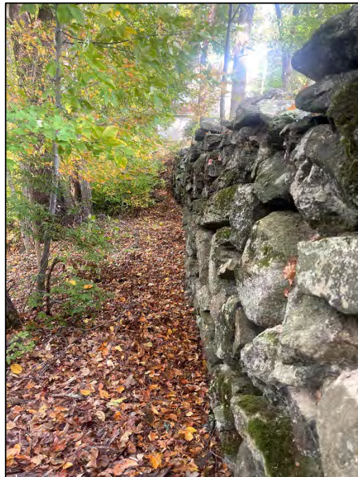
Photo No. 38.: West Dike - Downstream side as viewed from near STA D1+50 looking right. Note bulged stone wall.
