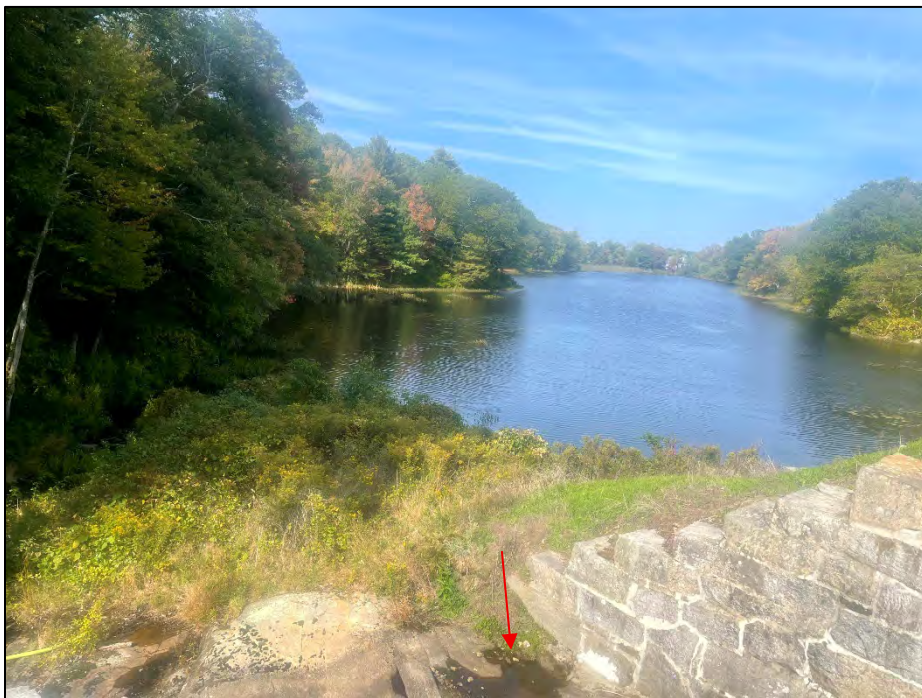
Photo No. 24.: Tailwater pond (Pascoag Reservoir Lower) as viewed from left of the primary spillway. Note clear leakage out of bedrock joint (arrow).
