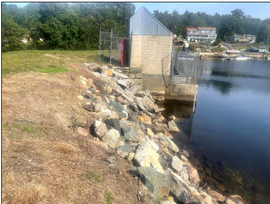
Photo No. 2.: Upstream slope as viewed from left of the primary spillway looking right. Note areas of thinning grass and bare surfaces along the upper part of the slope.
