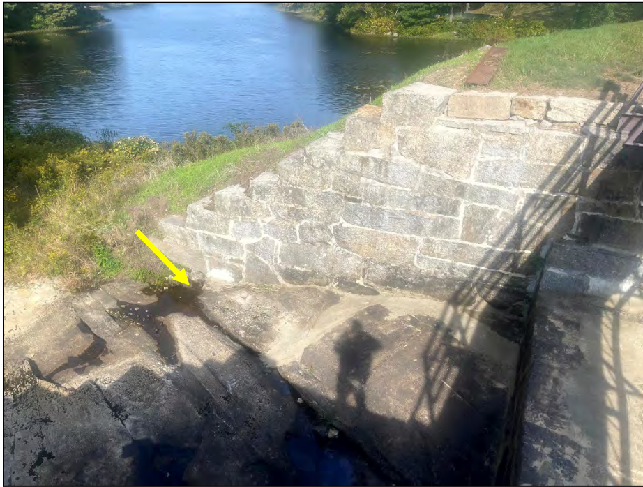
Photo No. 17.: Primary spillway downstream right wall. Note area of historic leakage (arrow).
