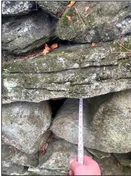
Photo No. 39.: West Dike - Typical gaps measured within the downstream stone wall. Photo of a 24 inch deep gap measured near STA 1+50.
