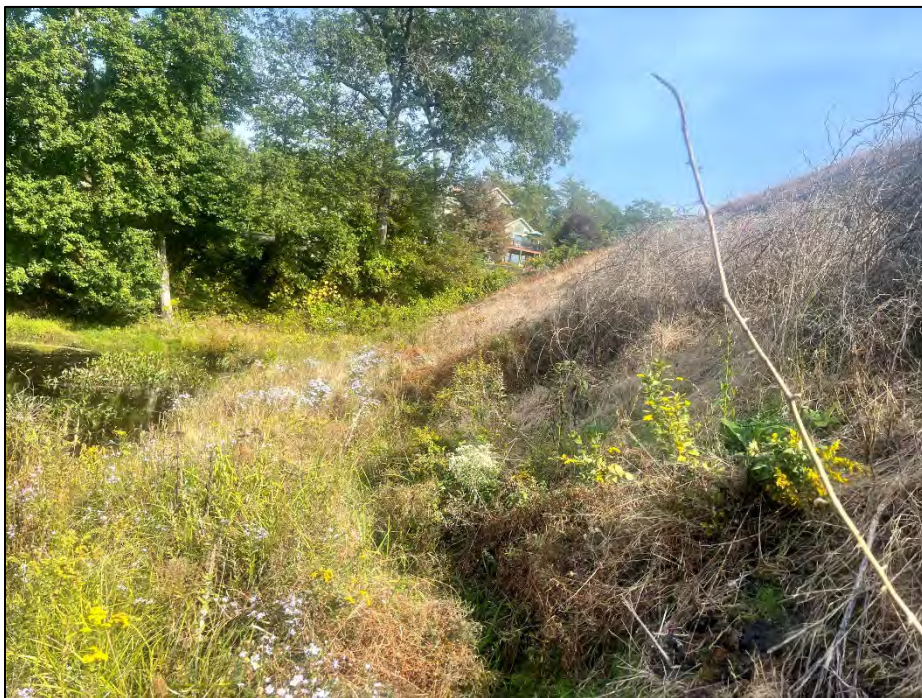
Photo No. 14.: Downstream slope as viewed from near STA 3+00 looking right. Note wet area along toe in the immediate foreground.
