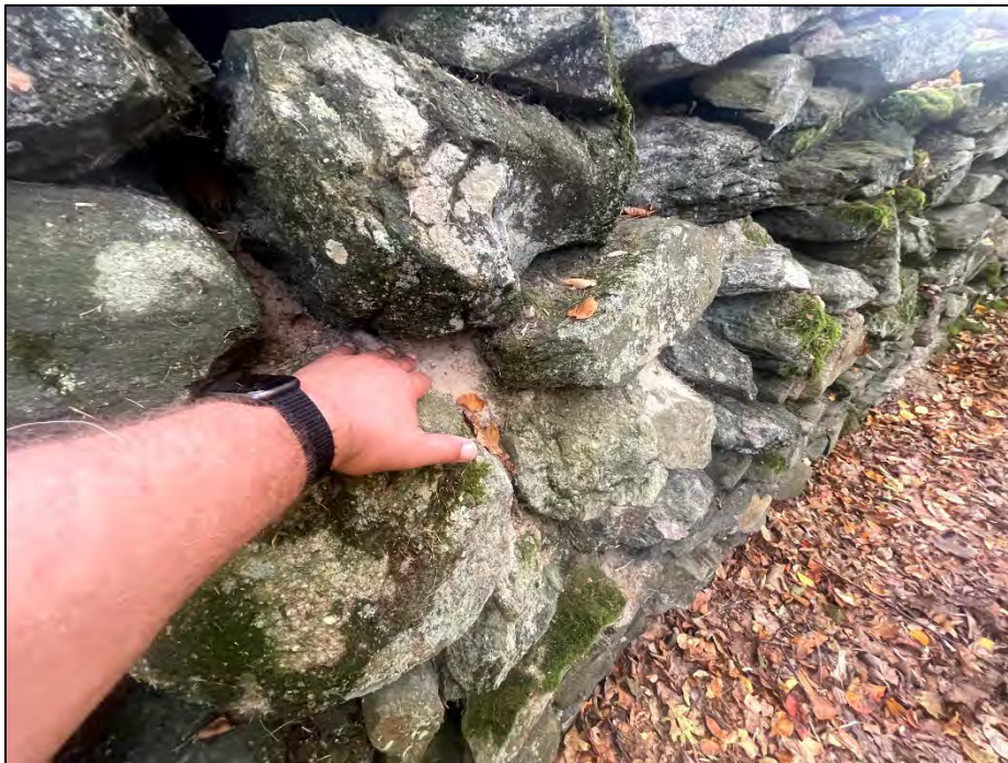
Photo No. 40.: West Dike - Sand discharge within gaps of downstream wall as viewed from near STA 2+00 looking right.
