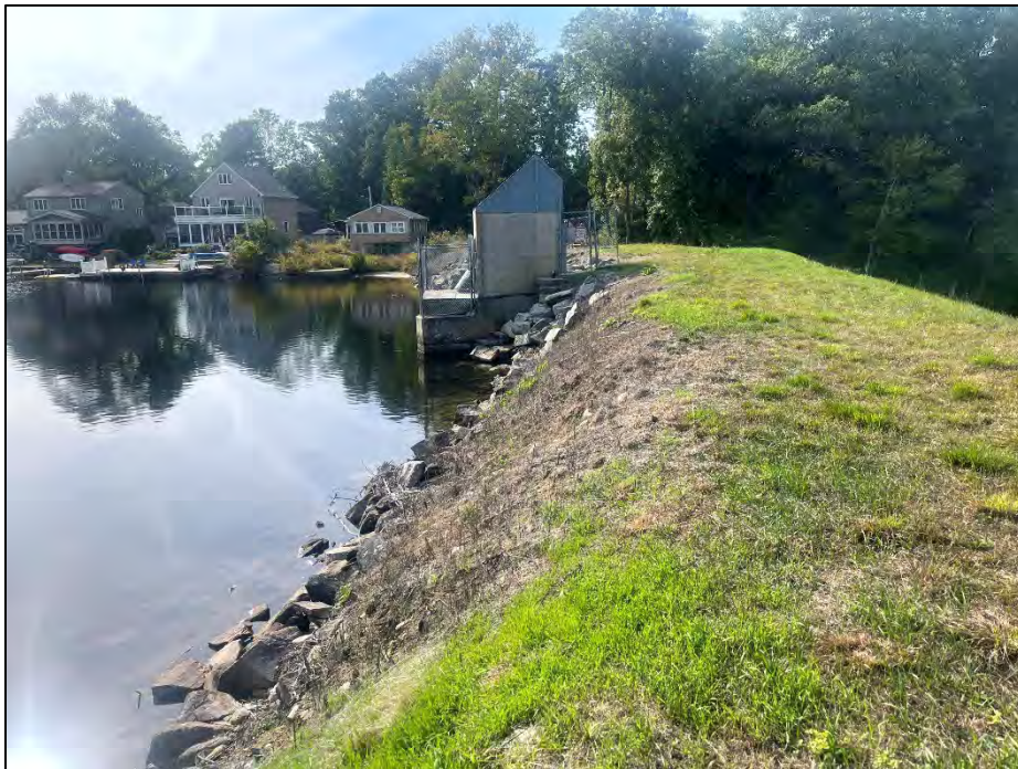
Photo No. 4.: Upstream slope as viewed from the crest near STA 2+60 looking left. Note areas of unraveled grass and shallow sliding failures.
