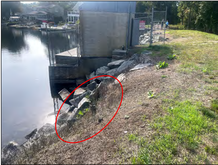
Photo No. 3.: Upstream slope as viewed from the crest near STA 2+00 looking left. Note area of shallow sliding failure (circle).
