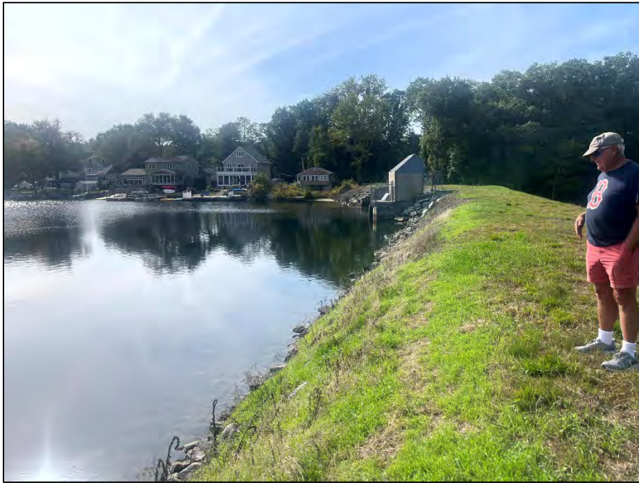
Photo No. 5.: Upstream slope as viewed from the crest near STA 4+10 looking left. Note typical steep slopes and sparse erosion protection.
