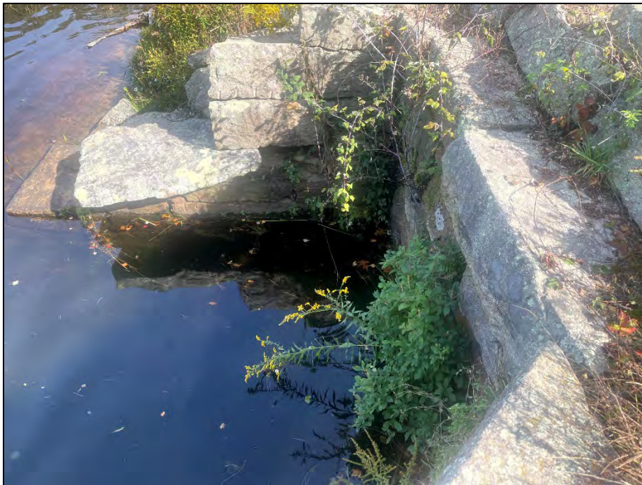
Photo No. 22.: Low level outlet downstream headwall. Note shifted wall stones and open joints, typical throughout the discharge structure.
